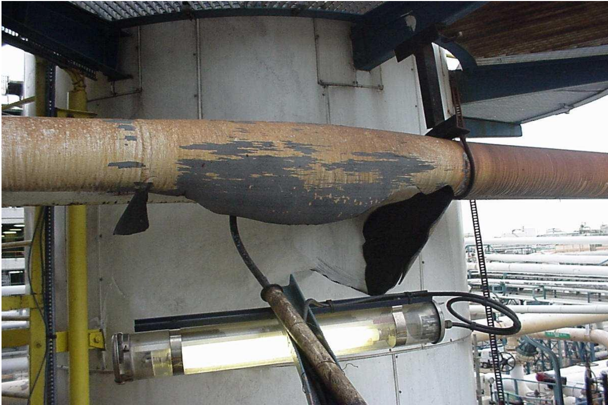
Figure 10. Pipe rupture caused by popcorn polymer in a butadiene unit in the Lavera petrochemical complex. (Credit: French Ministry of the Environment [12, p. 157])
