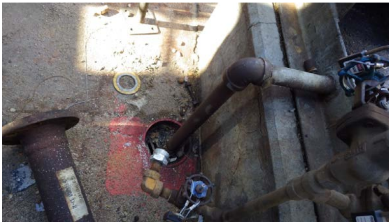
FIGURE 8. Typical pump drain to OWS (Source: CSB).
