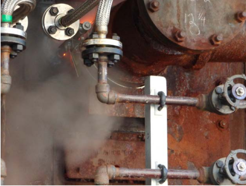
FIGURE 7. Burner on furnace (Source: CSB).
